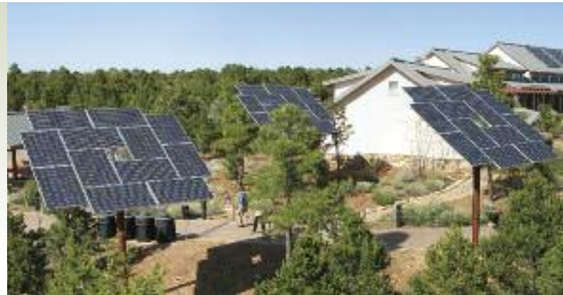
New solar panels at Grand Canyon National Park Visitor Center.
